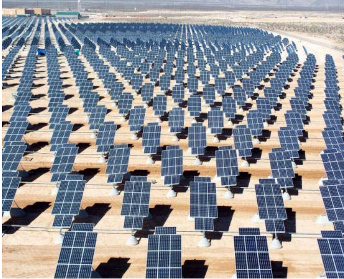
Figure 6: The Largest PV farm in the US, at Nellis Air Force Base in Nevada. At an output of 14.2 megawatts, it is exceeded in size and output only by the Photovoltaic Farm in Jumilla, Southern Spain (“Air Force base”).
